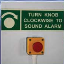
Internal panic alarm
