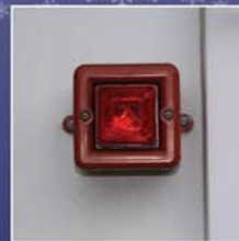
External panic alarm / beacon
